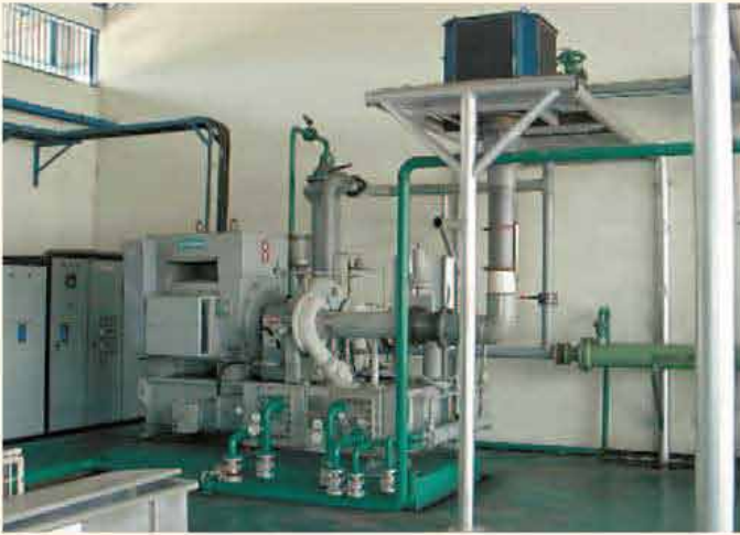
A 3,030 CFM (5,150 m 3 /hr) industrial air compressor. This compressor is installed in a manufacturing facility located in Indonesia.
