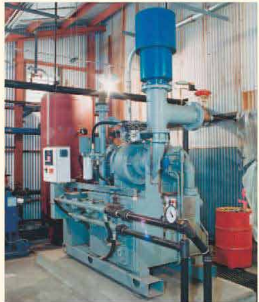
A 1,500 CFM (2,550 m 3 /hr) industrial air compressor with "D" flange mounted motor, being used in a steel mill.
