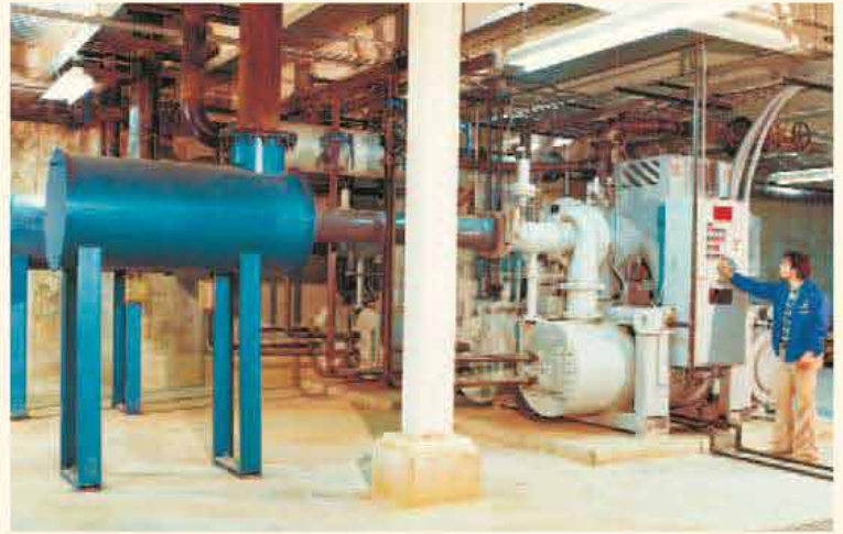
Two 4,200 CFM (7,140 m 3 /hr) PAP PLUS compressors supply 45 psi (3.1 bar) gage discharge pressure air to a glass manufacturing process.
